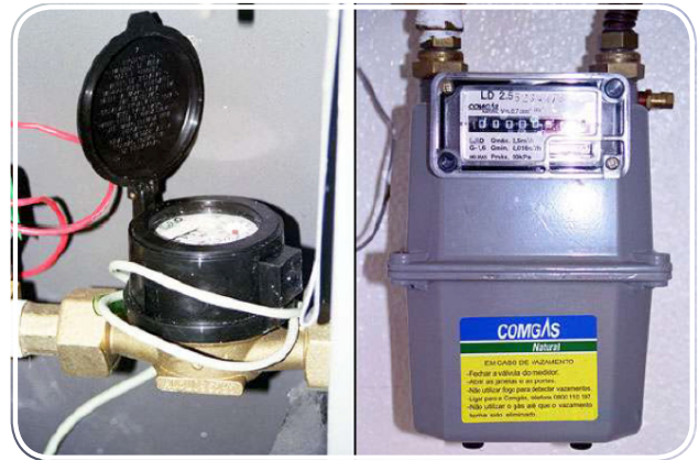
Figure 18 - Individual metering system with PLC technology in the CDHU's Mooca development. Source: QUALIHAB (2005)
