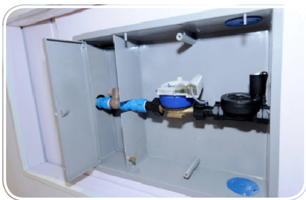
Figure 24 - Remote individual metering system in the Francisco Morato housing development. Source: MOBIX S.A. (2010)
